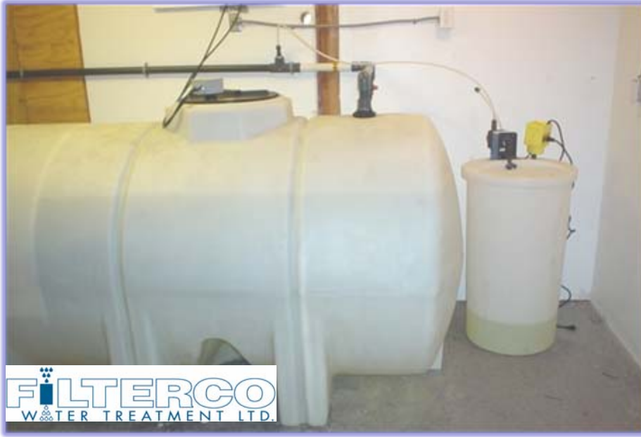
Hyper-chlorination with Contactor
