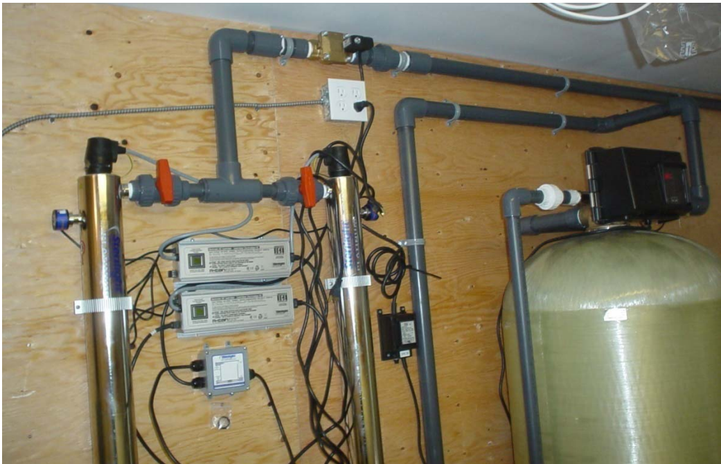
Automatic Filtration and duplex NSF-Rated UV Sterilizers c/w Solenoid Shut-Off
